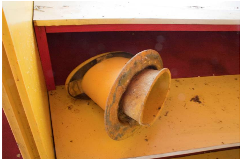
Figure 89. Protective cap of the air outlet has fallen down from the roof.
