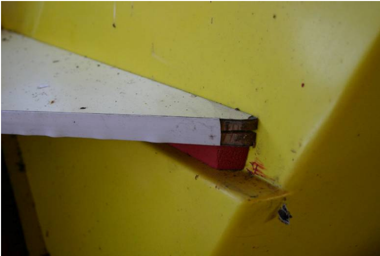
Figure 120. Missing part of the edging strip.
