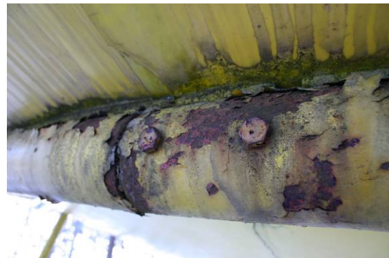
Figure 91. Corroded steel ring.
