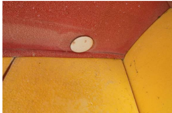
Figure 64. Air outlet in the ceiling.
