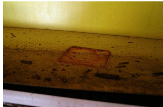
Figure 116. Rusty stains on the surface of the shelf.
