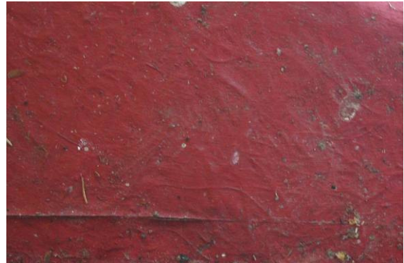
Figure 39. Uneven interior surface.
