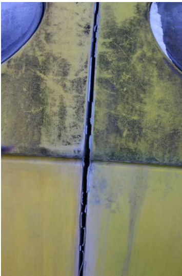
Figure 88. Many gaskets are cracked.
