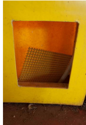
Figure 121. Loose grating on the ventilation hole.
