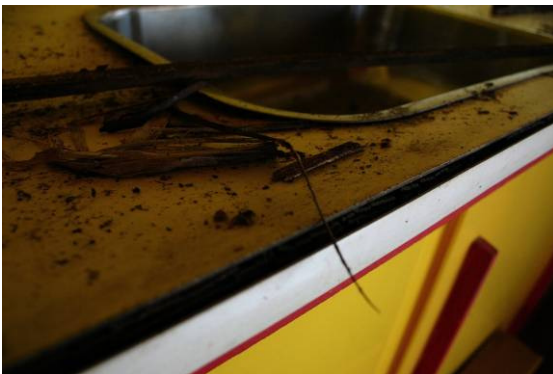
Figure 115. Loose edging strip.
